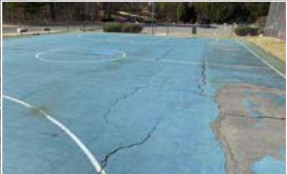
BASKETBALL COURT SURFACING IS IN NEED OF REPAIR
