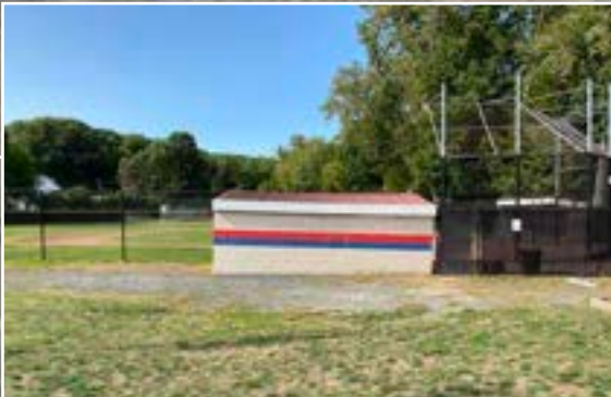
DUGOUT IS SETTLING
