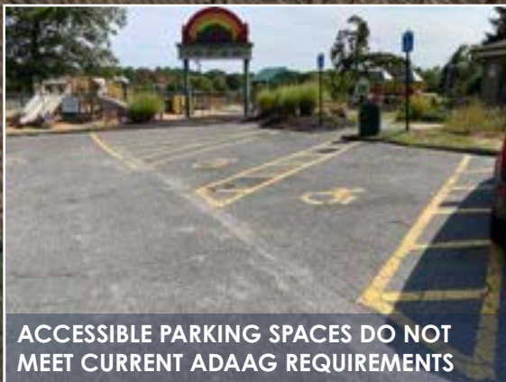
COURT ASPHALT AND SURFACING IS IN NEED OF REPAIR
