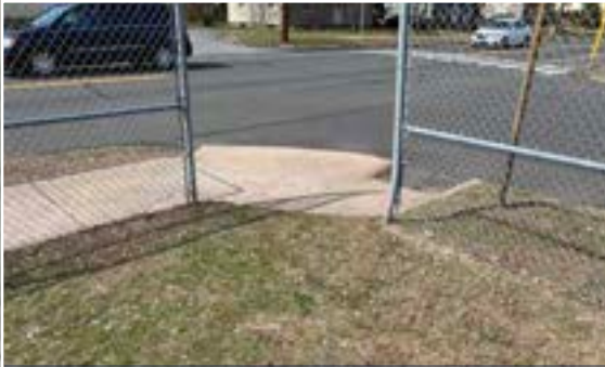
CURB RAMP DOES NOT MEET ADAAG REQUIREMENTS
