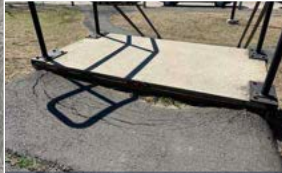
SETTLEMENT OF ASPHALT AT CONNECTION TO STAIRS LEADING TO OVERLOOK
