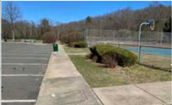
WALKWAY CROSS SLOPES TOO STEEP, CURB RAMP NOT UP TO CODE
