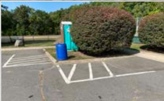
ACCESSIBLE CURB RAMPS AT PARKING SPACES ARE NOT UP TO CURRENT CODE
