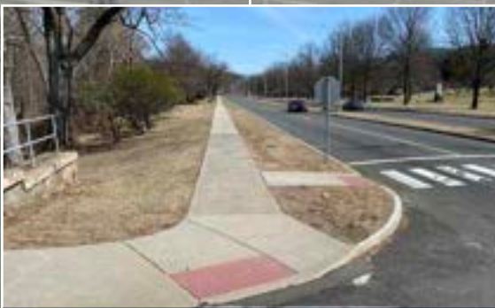
CURB RAMPS DO NOT MEET ADAAG REQUIREMENTS
