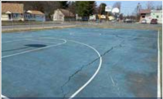
BASKETBALL COURT IS CRACKING AND REQUIRES REPAIR AND RESURFACING
