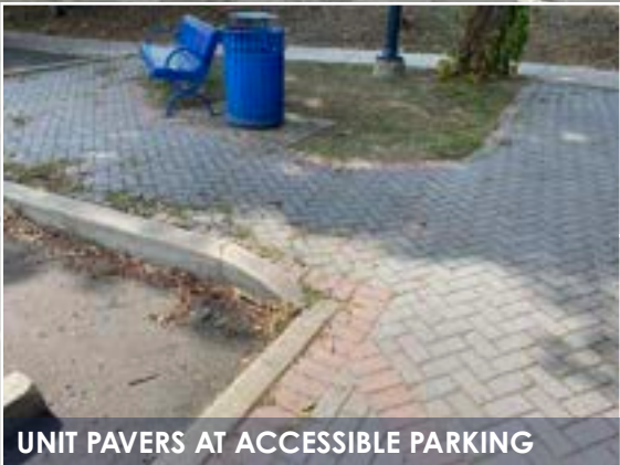
UNIT PAVERS AT ACCESSIBLE PARKING SPACES HAVE SETTLED AND AREN'T FLUSH
