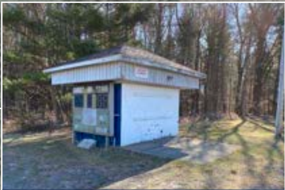
BUILDING IS IN NEED OF REPAIR
